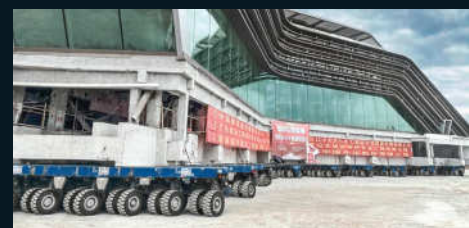
Sinotrans coupled the self-propelled SPMT platform transporters from TII SCHEUERLE at different angles to each other.
