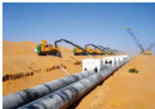
Borouge's Borcoat HE3450 is being used to coat sections of the 824 km pipeline.
