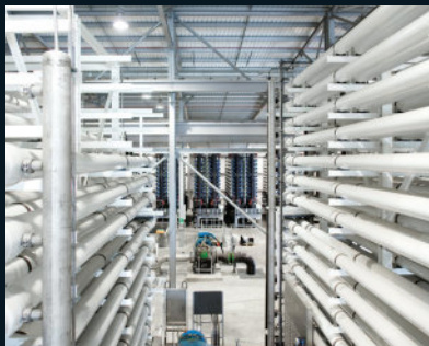
Once the plant is completed, ACCIONA will supply around 2.37mn m 3 /day of desalinated water in Saudi Arabia.
